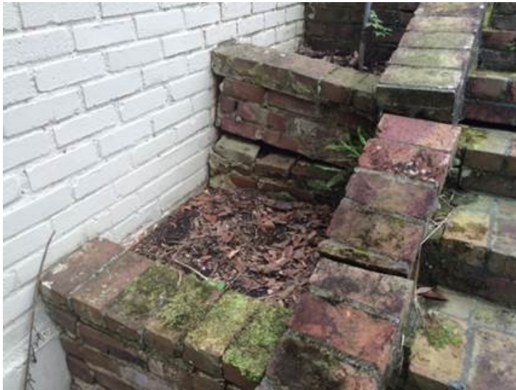
Broken Steps to Old Dorm Basement
