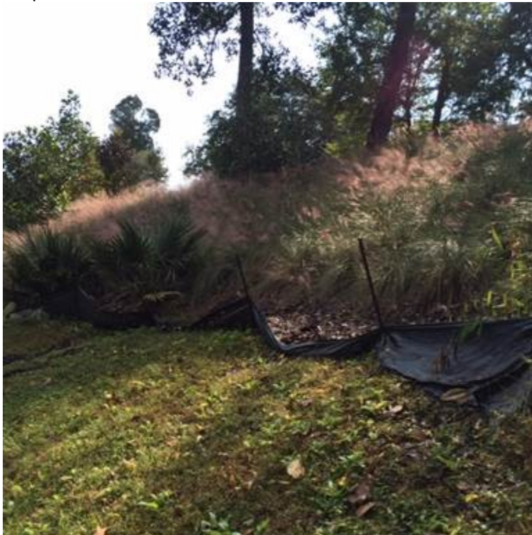
Silt fence damage at Columbarium
