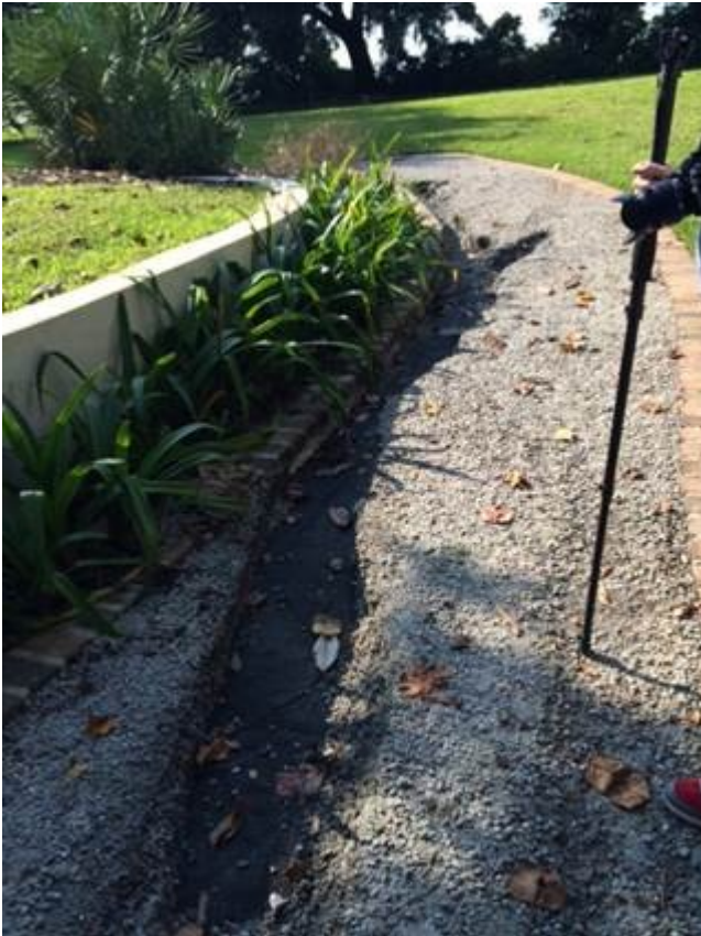
Path damage at The Columbarium
