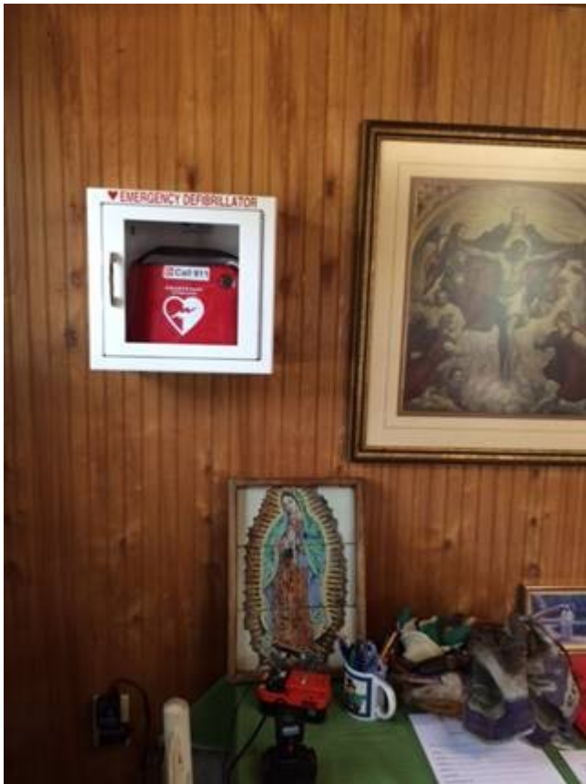
AED on left wall inside Breakroom
